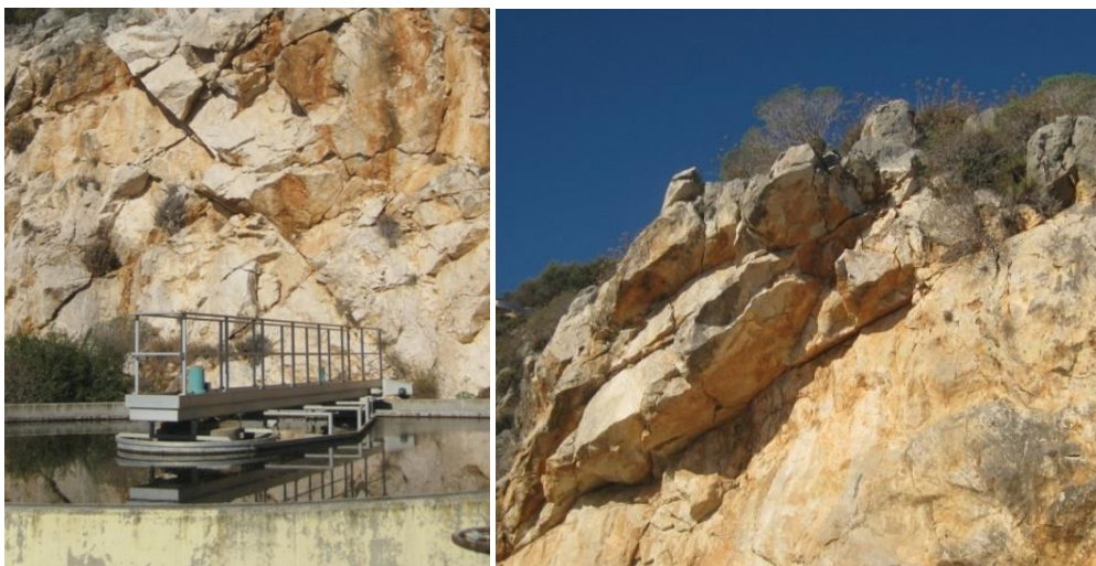
Figure 1: Left: Extended fractured rock slope close to one of the clarifiers of the facility. Right: Overhanging rocks.
