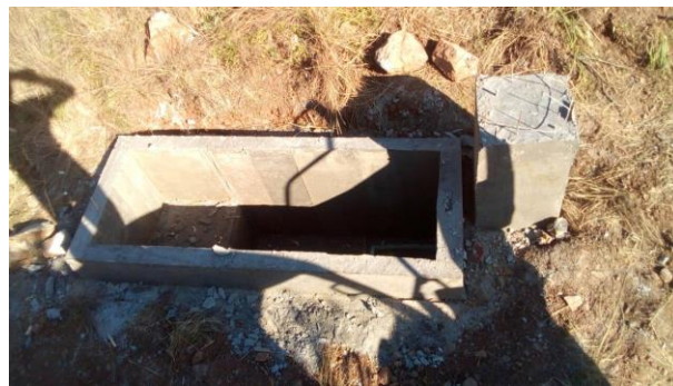
Figure 2. MET2 seismic vault under construction. The GNSS antenna will be installed on the concrete pillar.
