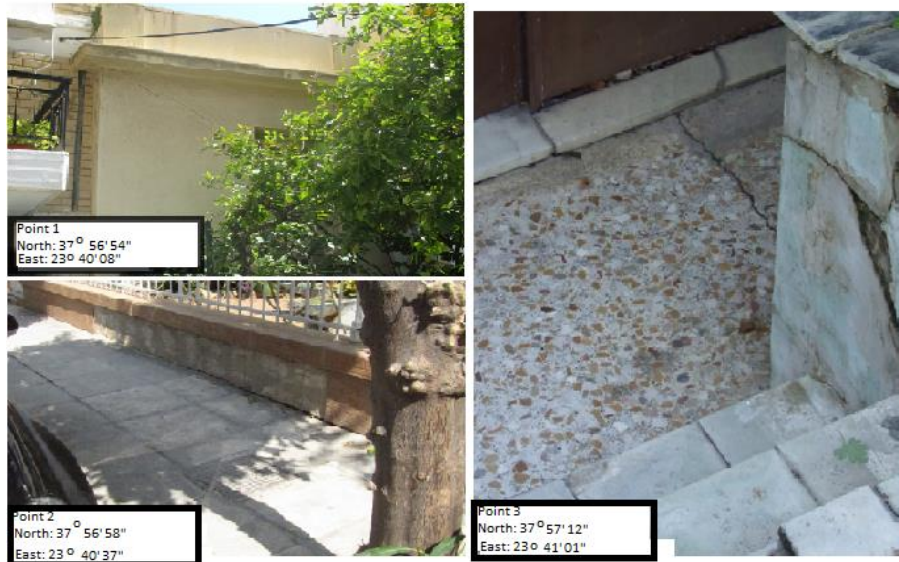
Figure 2. Field evidence of ruptures in the study area. Coordinates are in UTM WGS84 (projected). Damages witnessed at building (point 1), pavement (point 2) and natural terrain (point 3).
